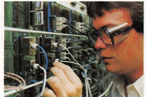
Engineer Colin Elliott checking out lightguide on the 3B processor.
