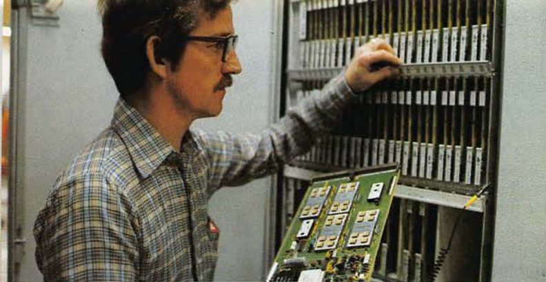
Installer Frank Reagan inserting gated diode circuit board in an Interface Module frame, heart of the local digital switch.
