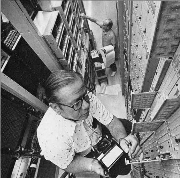
Bird's eye view of the first installation of T-1 Carrier, a digital or pulse-code modulation system for transmitting signals on inter-office trunks largely in urban areas.
