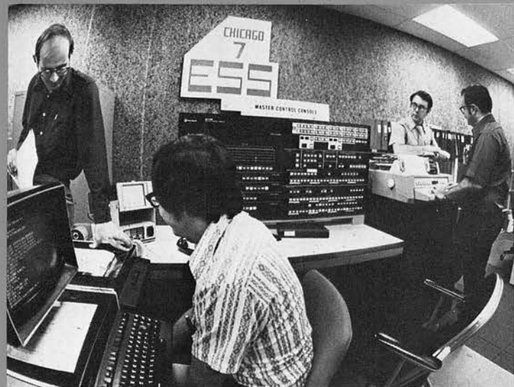
Western's electronic switching system for long distance calls, the #4 ESS, was our first digital switcher. The first installation was in Chicago. Rapidly, the 4E began to replace the #4 crossbar offices nationwide.
