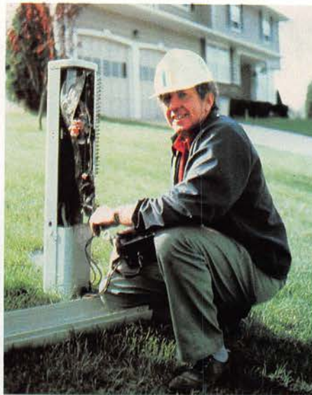
Your service lines are connected to a curbside pedestal.
