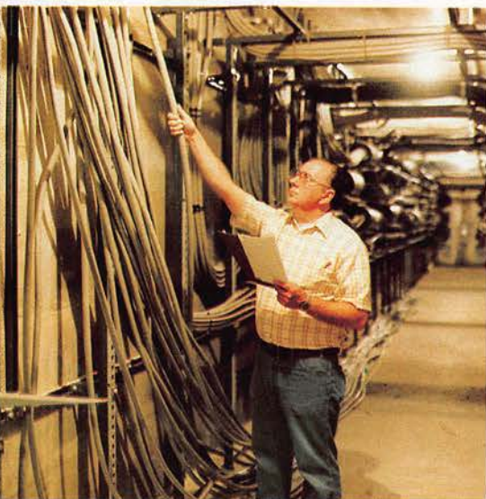
Incoming cables are connected to the central office's main frame.
