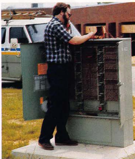
A distribution interface connects service lines to the exchange.
