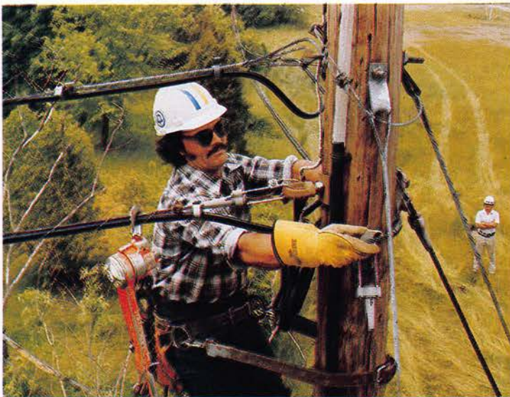
From high atop their enclosed cages, workers are either stringing cables or . . .
