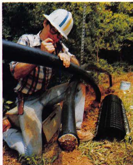
Loop cables are usually buried in the ground.
