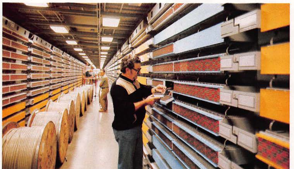
Cosmic II frames in central offices systematize the addition of new lines.
